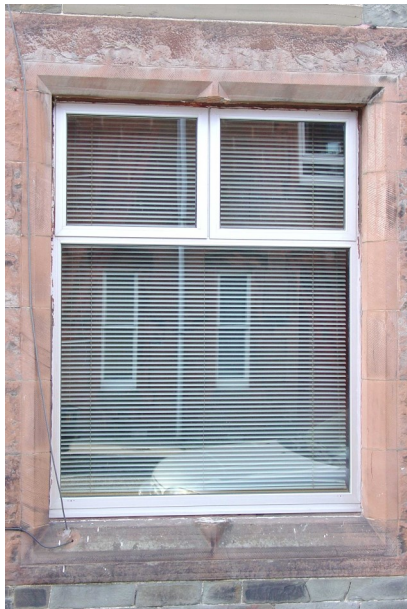
Figure 18: Replacement Window, which removes the central mullion and changes the whole character of the window opening.
