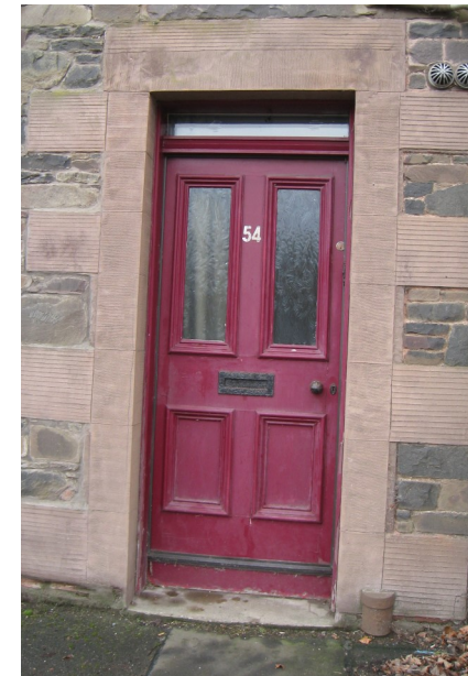
Figure 25: Door Alteration - Replacement of upper timber panels with glazing to allow additional light internally.
